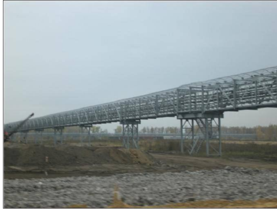
Cable Bridge for Electricity
